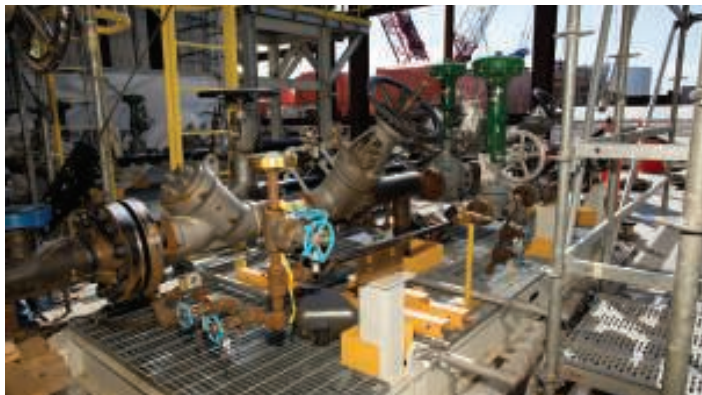
FIGURE 2. Input from operations and maintenance teams is required early on in the design process to ensure that modularized facilities can be easily maintained
