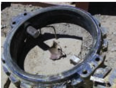
FIGURE 2. The iron disc of this seated butterfly valve was dissolved by sulfuric acid after the PVDF coating was removed by flowing acid
