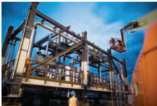
FIGURE 1. Modularization, the pre-assembly of structures away from the primary construction site, has many benefits, including improved labor productivity and reduced HSE risks
